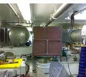
Figure 3.5: Urea tank in the aft ship.
